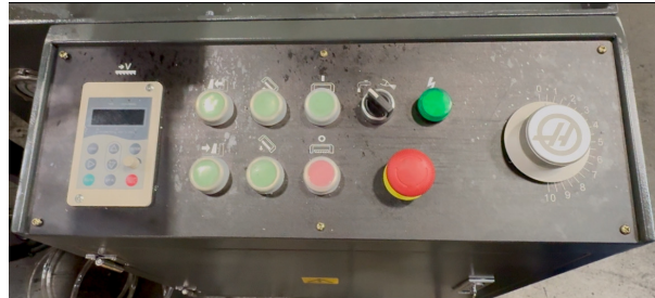
MAIN CONTROL PANEL
