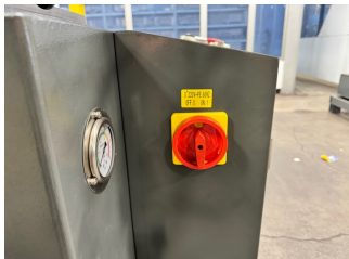
MASTER POWER SWITCH
