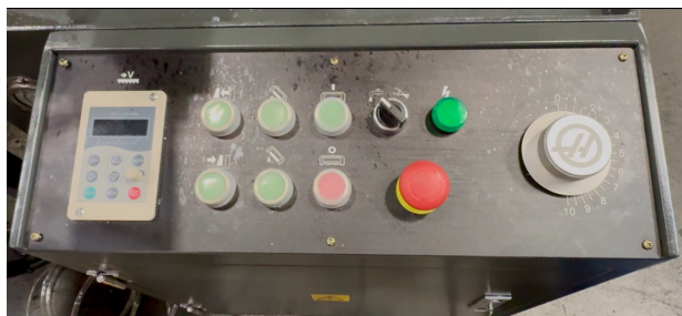
MAIN CONTROL PANEL
